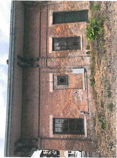
Photo A - Exterior Brick on Southeast corner of building
