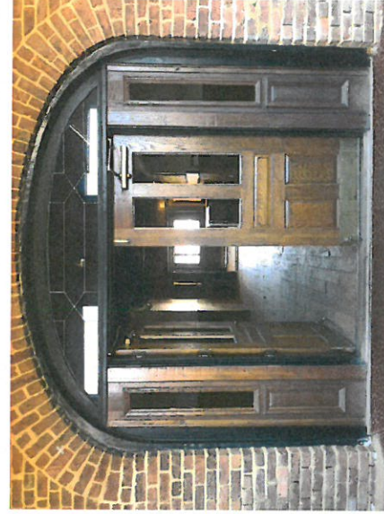
Photo F - Set of Doors from Lobby to be replicated in matching arched openings
