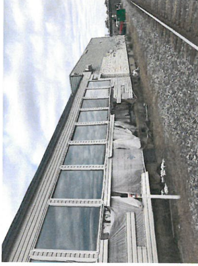
Photo C - Close up of damage on enclosed porch
